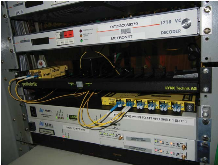
yellobrik fiber receivers and multiplexers at WKRN-TV Broadcast Facility
